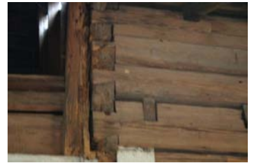
Detail of log notching on front of Hawthorne house visible under collapsed front porch
